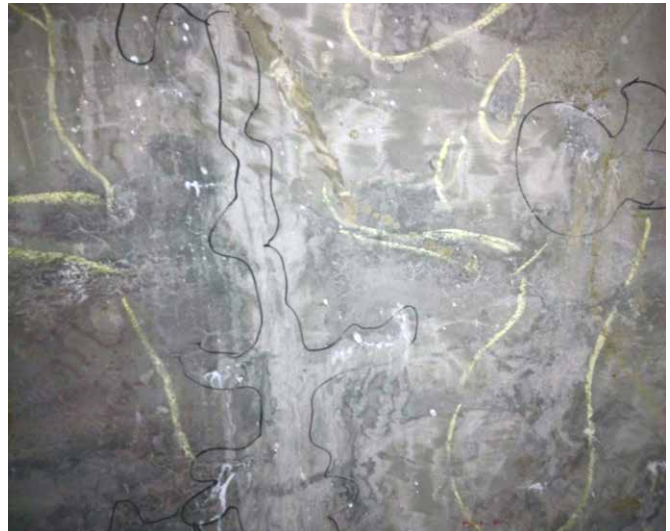
March 2012 – Cracks Healed
