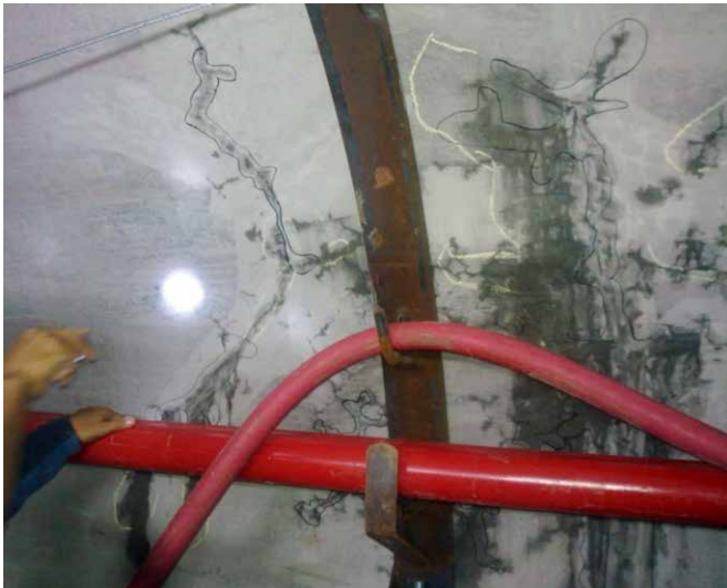
November 2011 – Weeping Cracks
