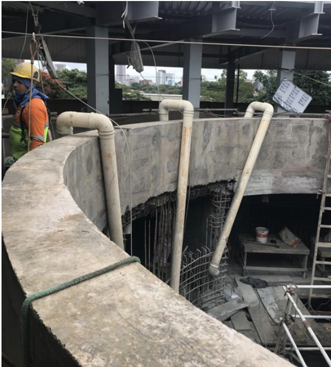
A view of concrete treated with Xypex Bio-San at the Pinheiros sewage pumping station, ensuring protection against microbial induced corrosion.
