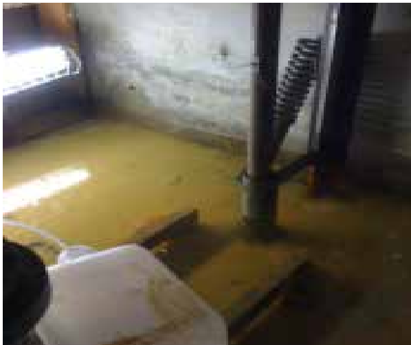
Water Ingress in Elevator Pit
