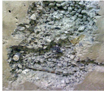
Construction defects (rock pockets, honeycombs & untreated tie holes)
