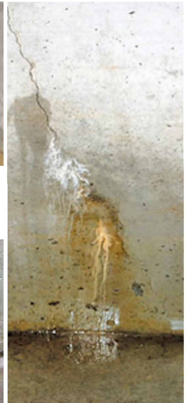
Leaking through cracks / joints
